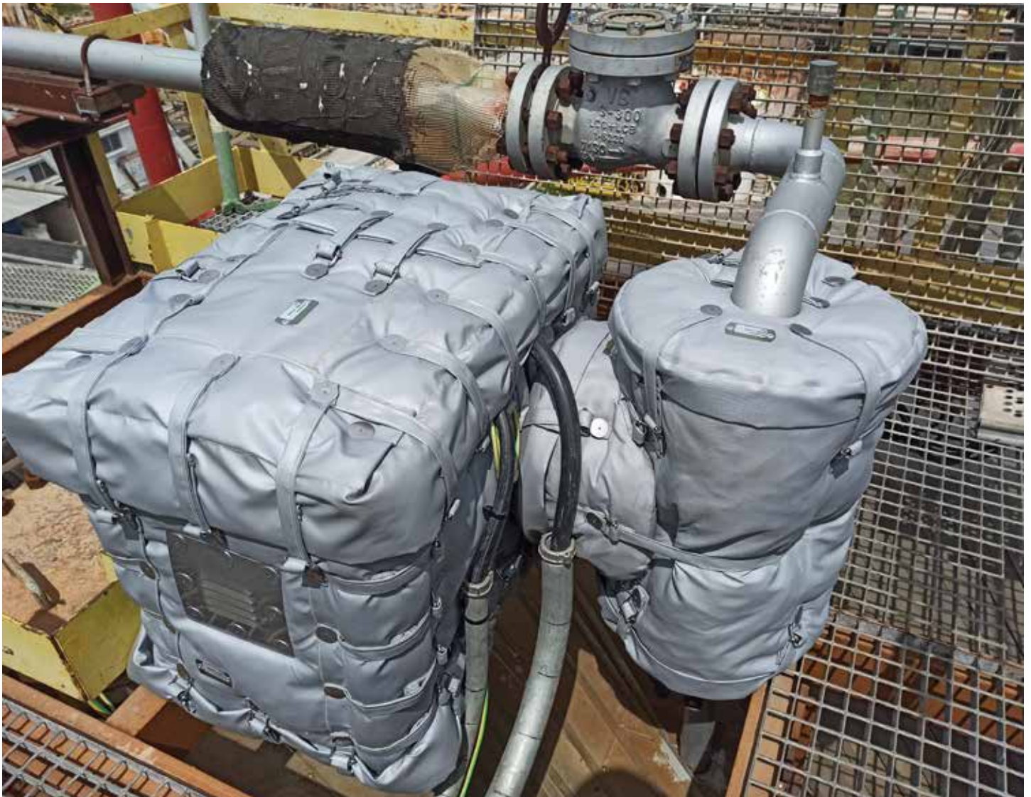
Flexible PFP on actuated valve
