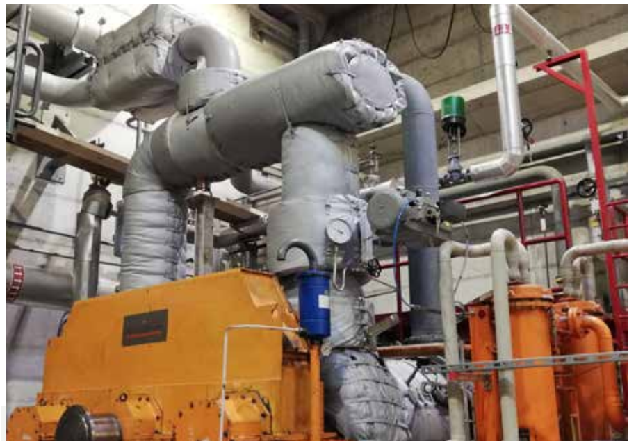
Piping and turbine
